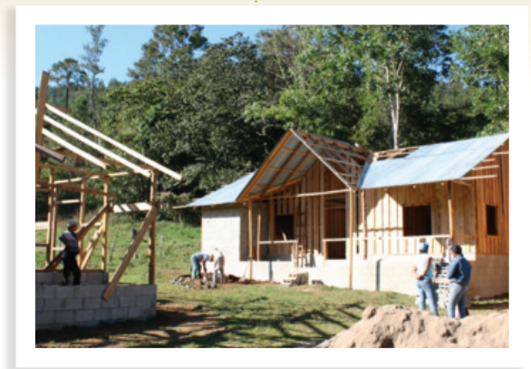
Cabin construction is on its way! 95% of construction materials were purchased last quarter.
